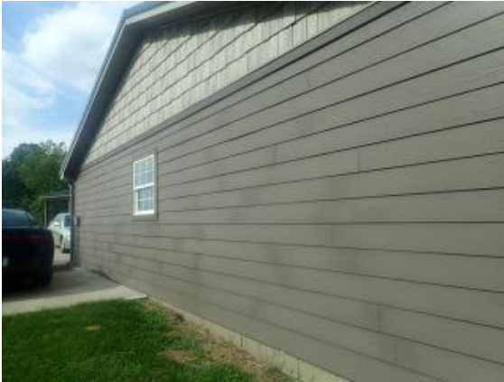
Faded Paint and Repairs noted along south side of Garage.
